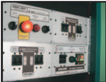
Power Distribution Modules
